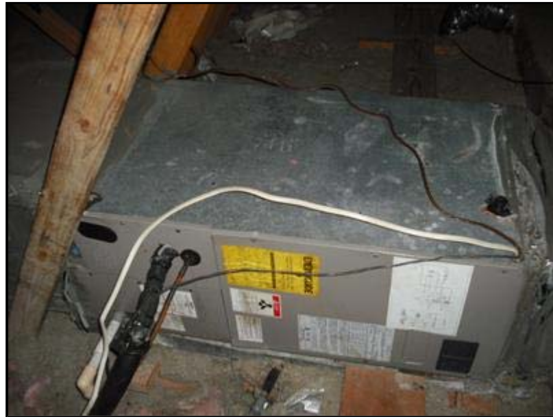
Air Handler Attic
