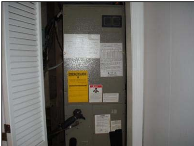
Air Handler 1st floor
